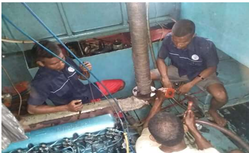
Figure 2. Main Engine MITSUBISHI 160 PK
