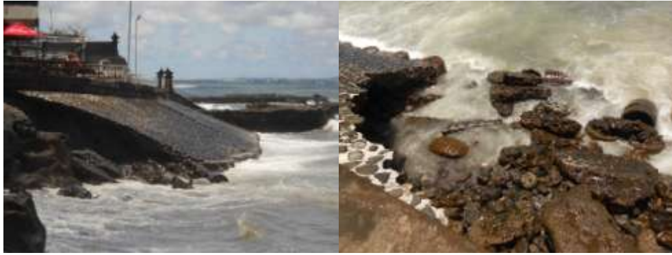
Figure 1 Coastal Protection Work damage at BatuMejan Beach
