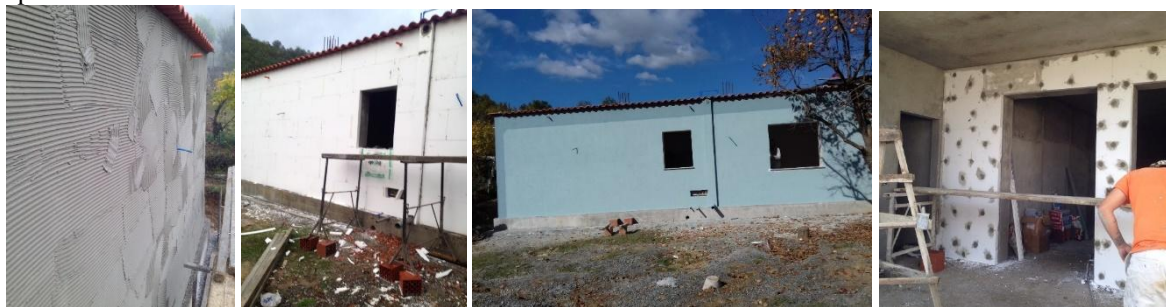
Figure 7. Villa in the village of Burel. During the placement of the thermal insulation material; source: Luca Ndertim[7]
