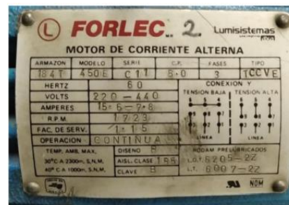
Fig. 14. Motor under test data plate
