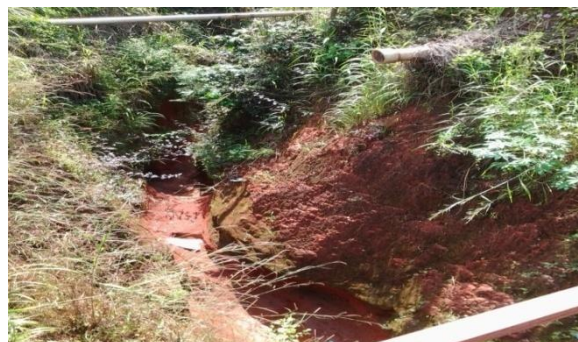
Fig 2: A gully at Uruegbe with a water pipeline destroyed
