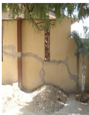
Plate iii: cracks on the wall
