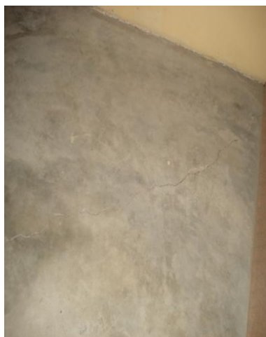
Plate v: Cracks on floors
