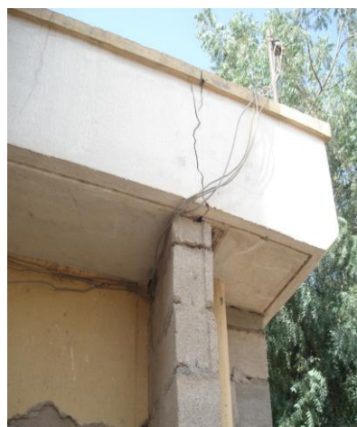
plate vi: cracks on parapet wall
