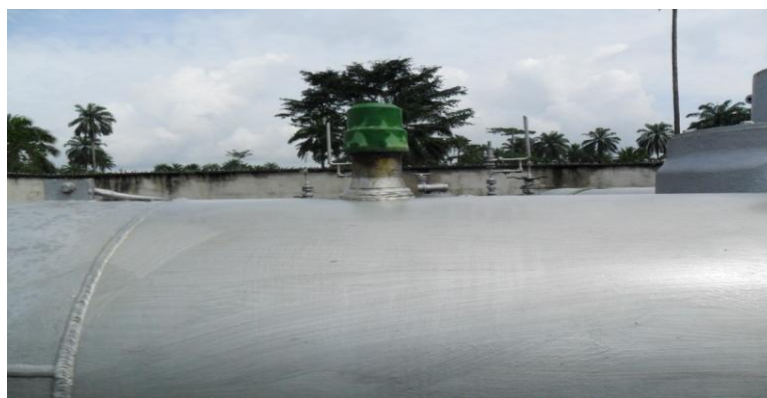
Plate 2: Access valve for insertion of coupon in a 24" pipeline.
